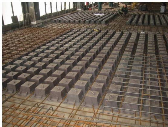
Fig. 4 Reconstruction of Skoda factory hall in Mlada Boleslav – composition of waffle fillers from RMWP on existing floor structure
